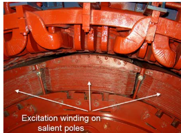
Fig. 6. View on the rotor of the generator in Hydro Power Plant HE "Vinodol" ( o = 40 )
